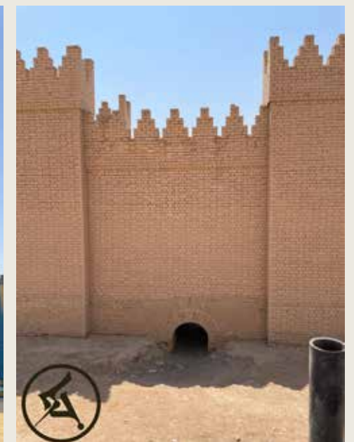
A prime example of the damage wrought upon Babylon's ruins by Saddam's vanity project. The best way to tell if the portions of the walls are original is by the obvious darker hues at the base of the wall. According to the archeologist, these portions of the walls cannot be further excavated due to the weight of the new bricks on top. In fact, here lies one of the narrower gates of Babylon, forever buried underneath by Saddam.
