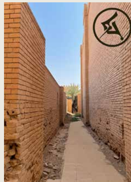
One of the many narrow corridors in Babylon. This one well exemplifies the impoverished state of the original bricks of Babylon holding up the weight of the newly laid Saddam-era bricks.
